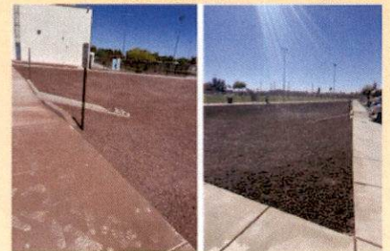
Rock was installed at the Joe Orduño basin west side of the soccer field.
