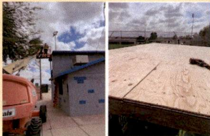
Roof and announcers' box was repaired at the Joe Orduño snack bar.
