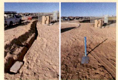
A new 3" water line was installed at the East Community Park for future sport field.
